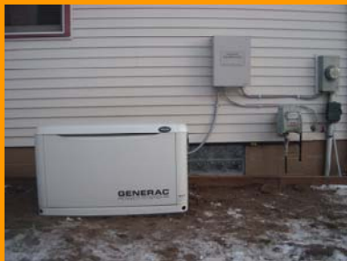
14 KW Generac Stand Alone Generator with a 100 AMP Transfer Switch
